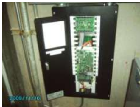
6 new relay panels were installed with new switching schedules that coincide with the school year schedule, including holidays off.
