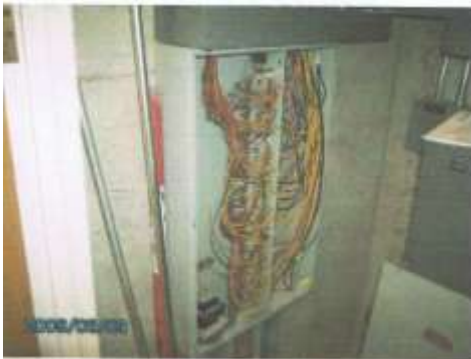
Existing controls system had failed several years ago.
